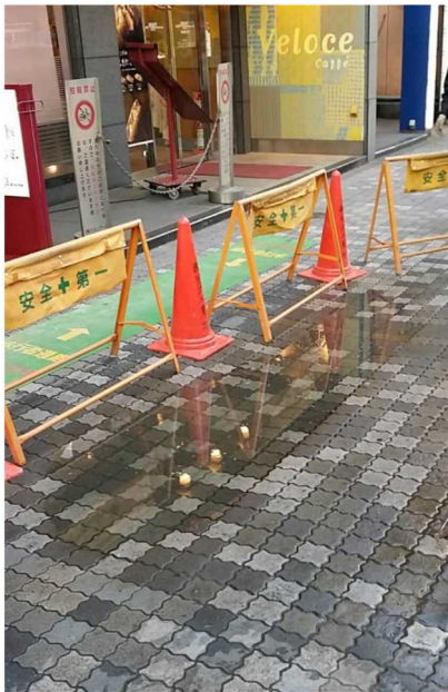
Fig.14 Service pipe leakage (seep through to the surface)
