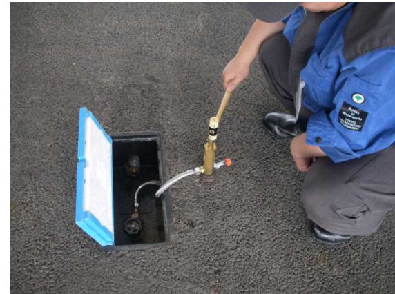
Fig.29 Water hammer Generator
