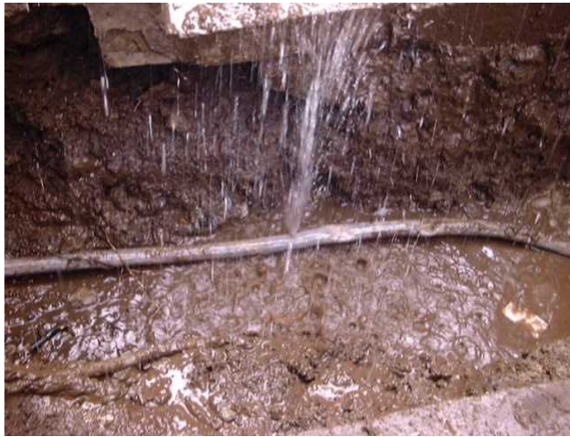
Fig.11 Leakage from lead pipes
