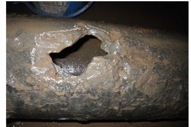
Fig.2 Corrosion leakage of iron pipes
