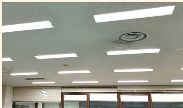
LED lighting (Misato Water Purification Plant)
