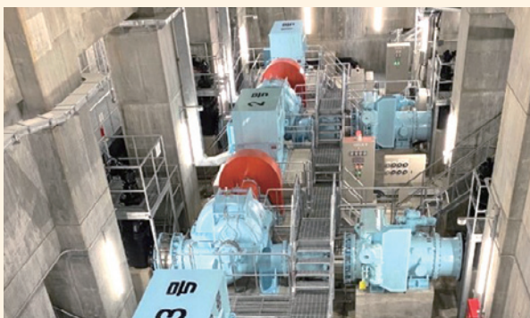
Energy saving pump equipment (Misumi Booster Pumping Station)
