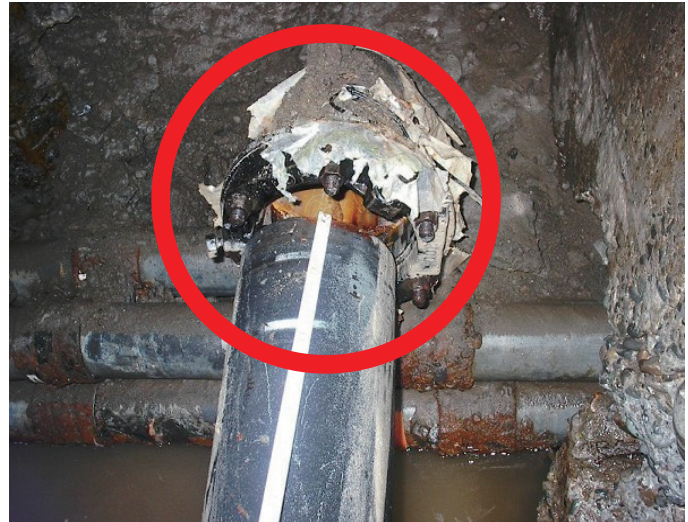
Dislodged pipe due to a lack of protective measures
