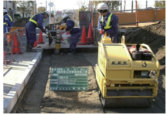
Compaction work performed by a roller and workers (Congested work is extremely dangerous)
