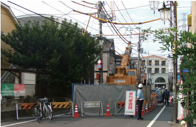
Overhead line protection
