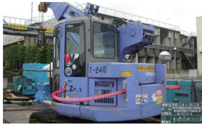
Backhoe contact prevention device
