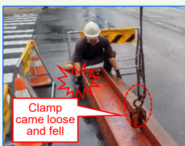
Injured while holding the bottom of an H-shaped steel member (FY 2022)
