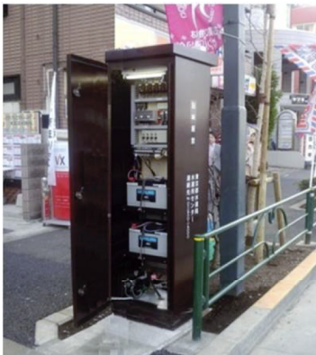
Figure 6 - Aboveground telemeter equipped with rechargeable batteries
