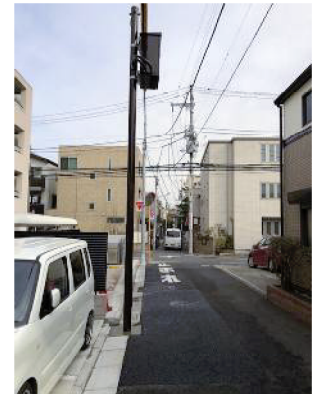
Figure 9 - Pole-mounted rechargeable batteries board
