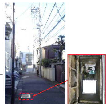
Figure 5 - Picture of Underground Telemeter
