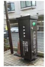
Figure 1: Telemeter board exterior
