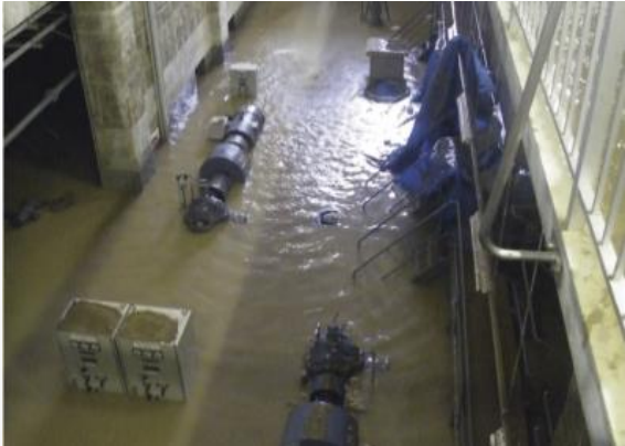
Pump room flooding (Yamaguchi Pref.)
