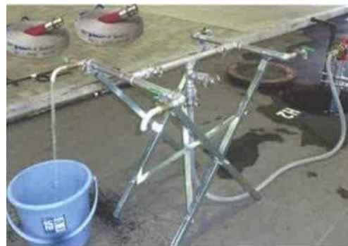
Figure 12 Emergency water supply when there is an earthquake
