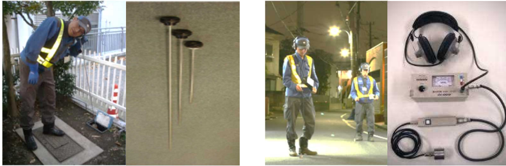
Figure 6 Acoustic inspection using sound detection bar (day) and using electronic water leakage detector (night)
