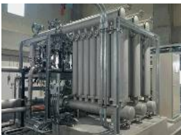
Figure 6— Membrane filtration equipment (inorganic MF membrane)
