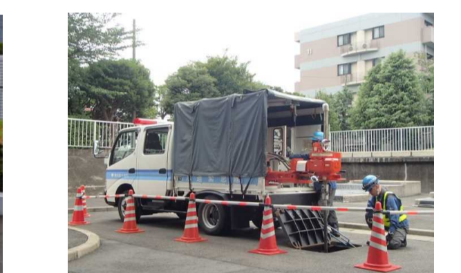
Gate Valve Operation Vehicle
