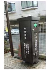
Figure 1: Telemeter board exterior
