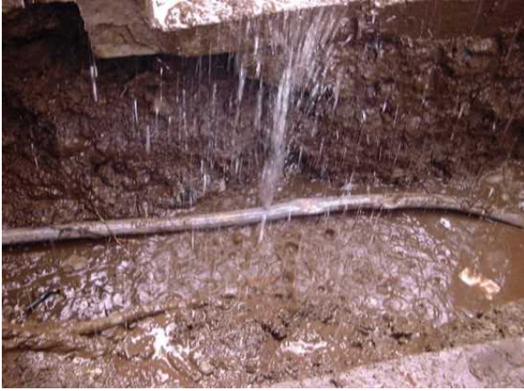
Fig.9 Leakage from lead pipes
