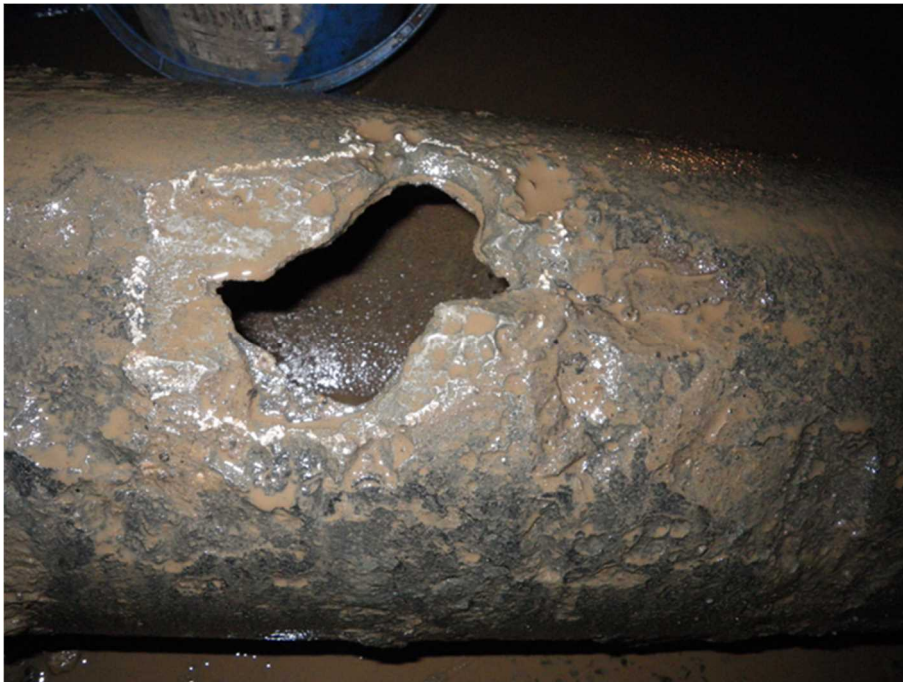
Fig.4-2 Corrosion leakage of iron pipes
