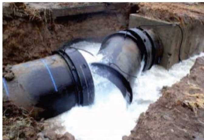
Photo 1 Damage on a Water Pipe in the Great East Japan Earthquake
