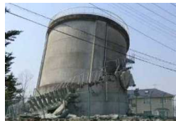
【Figure 2】 Damage example due to earthquake (Damage on a water tower)
